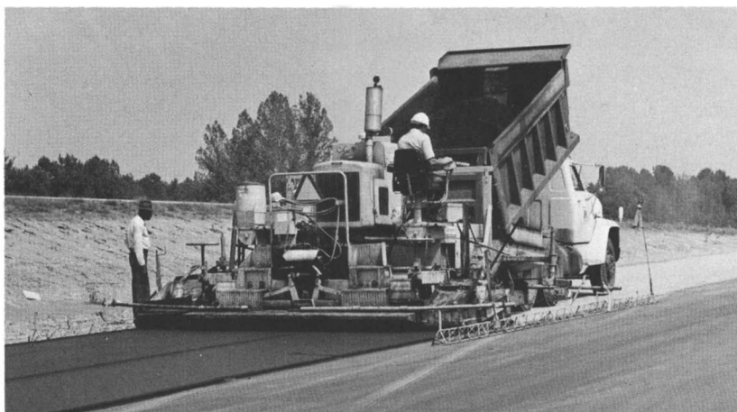
Figure 3. Conventional hot-mix paver and haul equipment used to place both the sulfur-asphalt and non-sulfur-containing mixes
